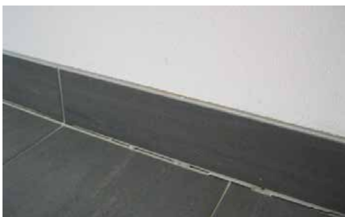
Fig. 23 – A cracked expansion joint without the use of a separation cord
