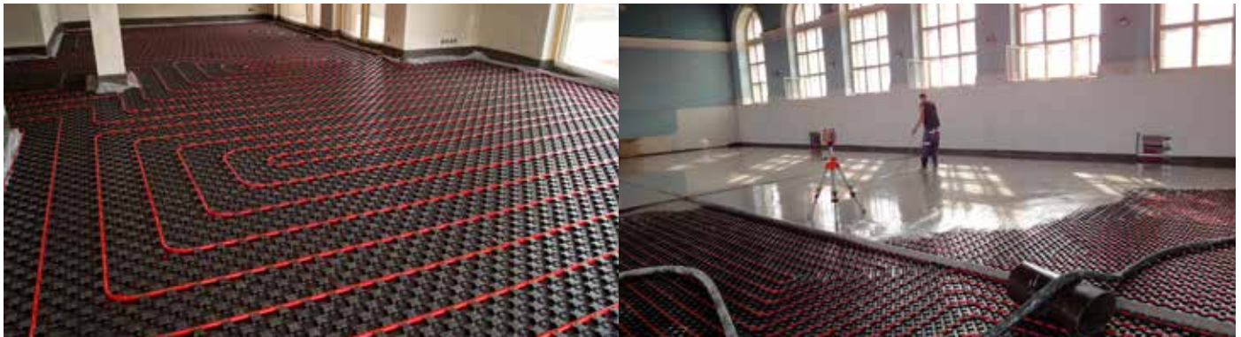
Fig. 16 – Example of water-based underfloor heating
