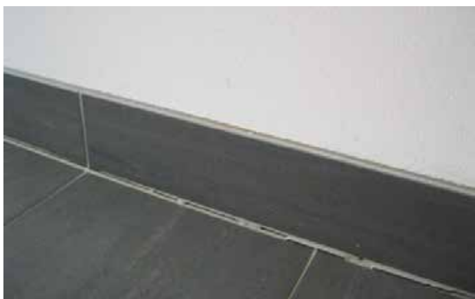
Obr. 23 – A cracked expansion joint without the use of a separation cord
